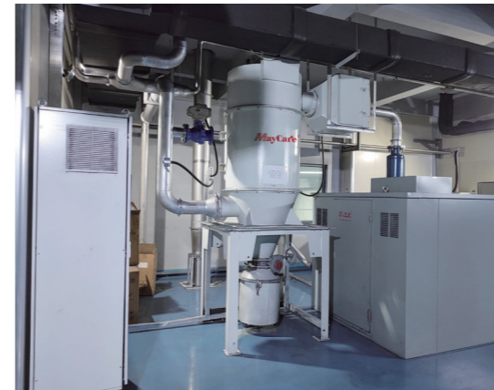
HIGH NEGATIVE PRESSURE DUST COLLECTOR Used for cleaning in lithium battery cathode material workshops
