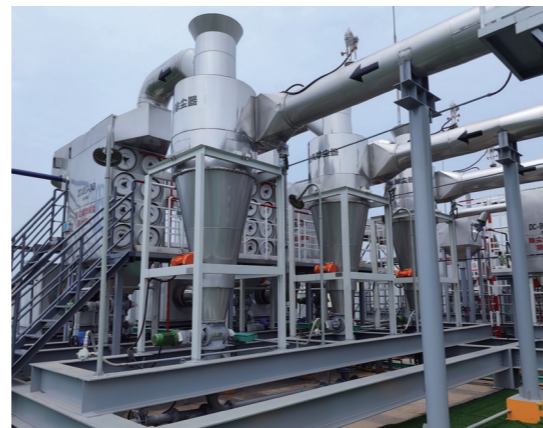
CARTRIDGE DUST REMOVAL SYSTEM Applied in the polysilicon industry
